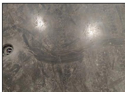
Figure 1 Cracks in Corundum Floor
