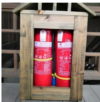
Figure 11 Indoor Fire Extinguisher Box Physical Picture
