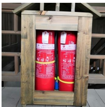
Figure 11 Indoor Fire Extinguisher Box Physical Picture
